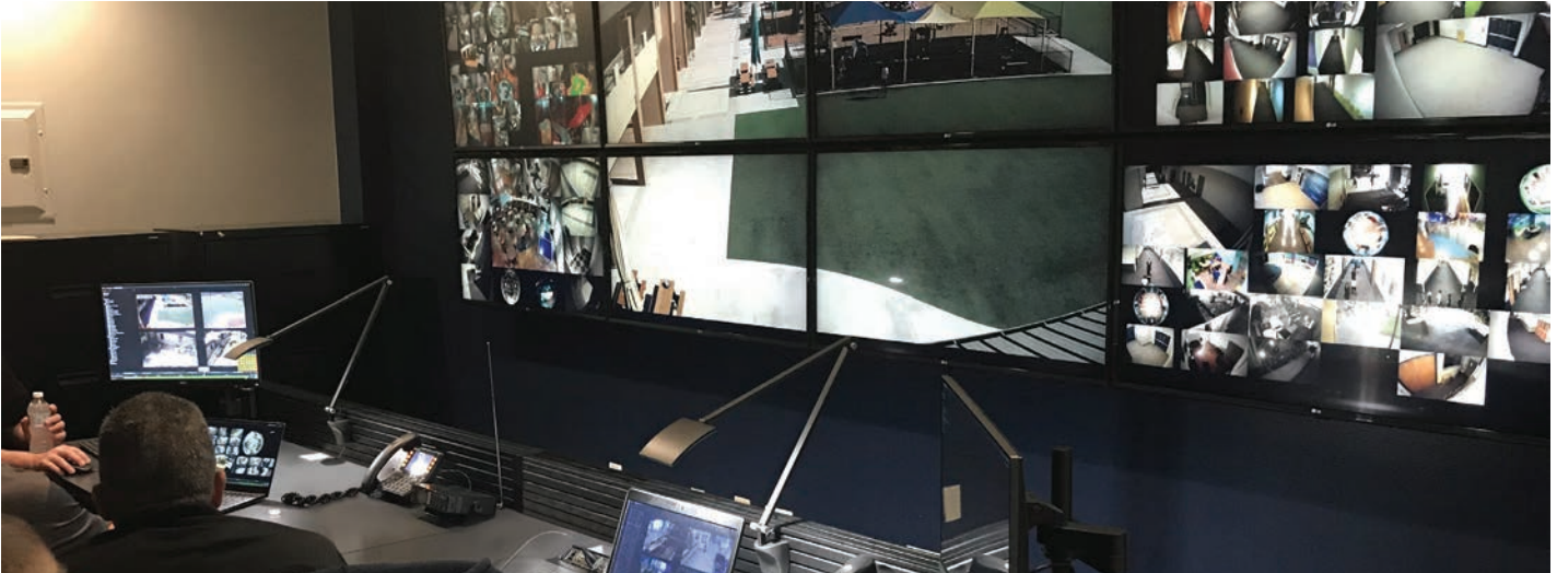
Video Wall users can create and remotely manage remote monitors with just a few clicks.
